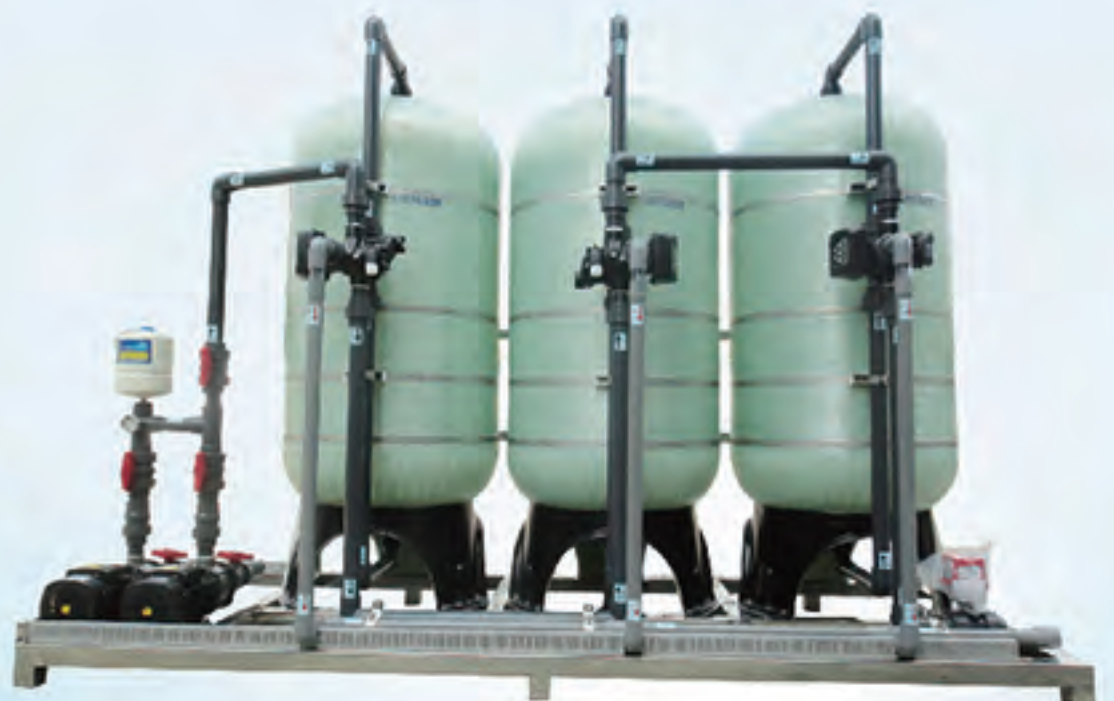
Whole pretreatment system ( top& bottom )
